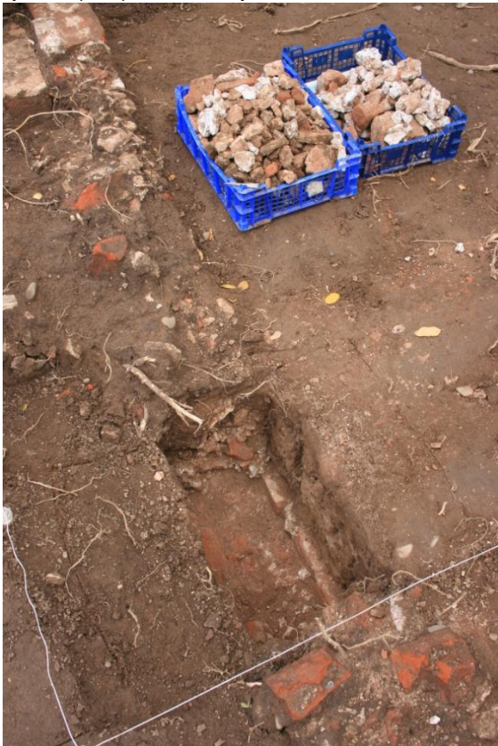
22. West wing, south/external wall 324, under excavation, showing part-buried external base course and the character of the rubble retrieved from the robber trench. Looking east.
