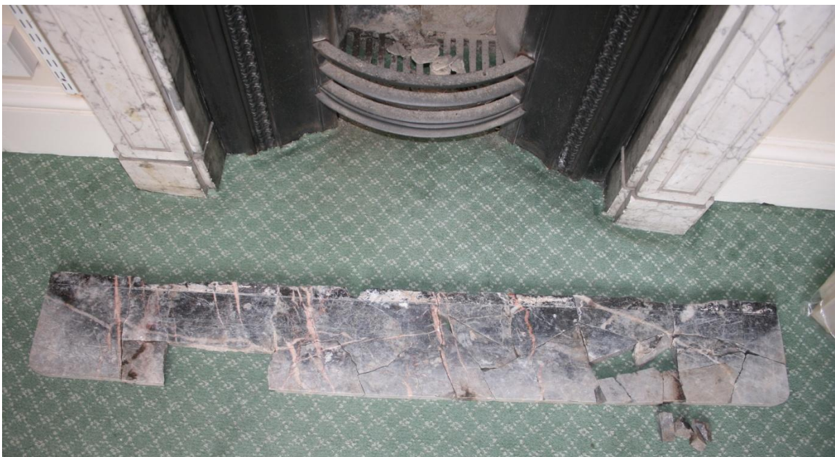
30. The mantelpiece reconstructed in front of a not entirely dissimilar fireplace in the Hub
